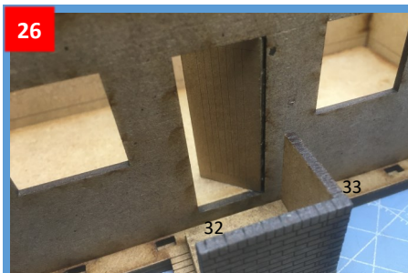
26 Glue the step walls (32 & 33) into position and the main door as preferred (shown open)
